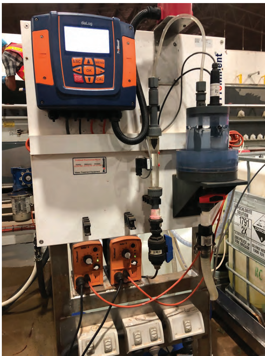
Figure 35. An automated chlorine injection and monitoring system.
