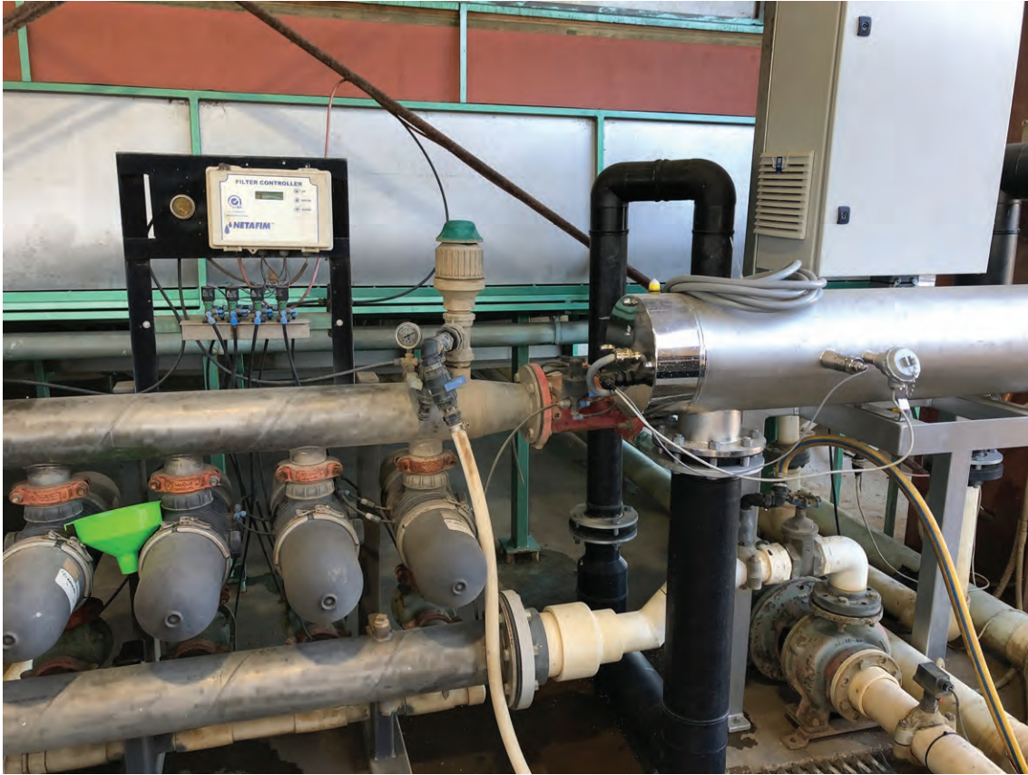
Figure 25. Wash water filtration.
