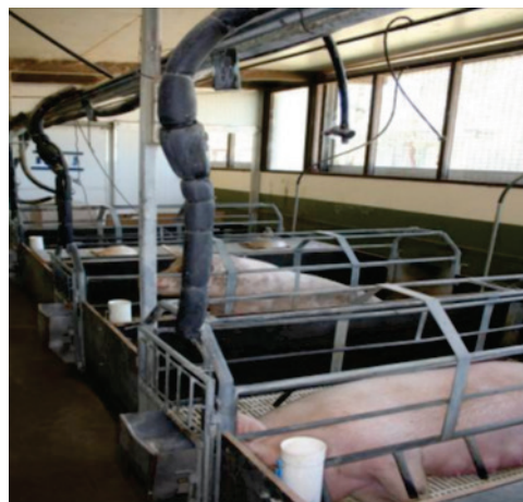
Figure 4: Water lines insulated with Supa-Ion refrigeration insulation.
