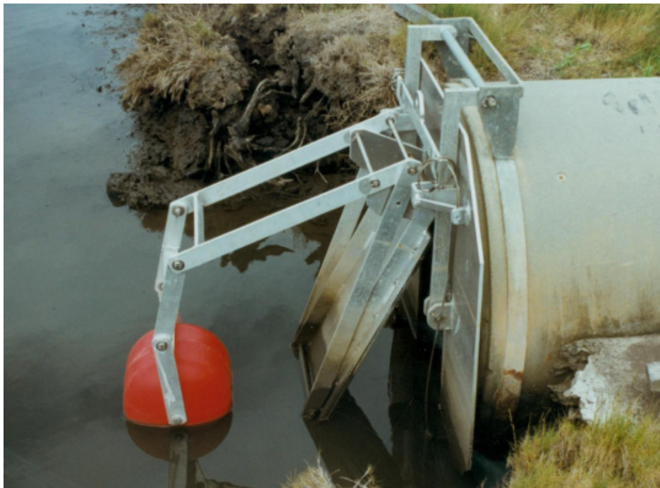
Figure 31 Tidal floodgate which opens and closes as downstream water levels lower and raise the float.
