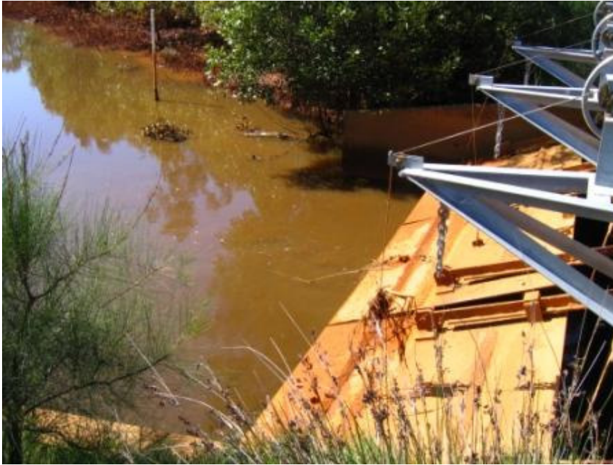
Figure 6 Wallis Creek floodgates and mangrove community coated in iron floc. (photo: A. Burke)
