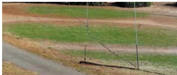
An example of a badly designed sprinkler system. A well designed system would have each wetting pattern overlapping to provide an even application.
