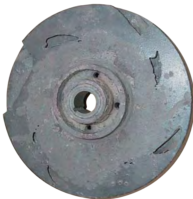
A badly eroded pump impeller. This can be caused through turbidity or through operating the pump outside its effective limits. It will increase energy costs and severely reduce capacity.
