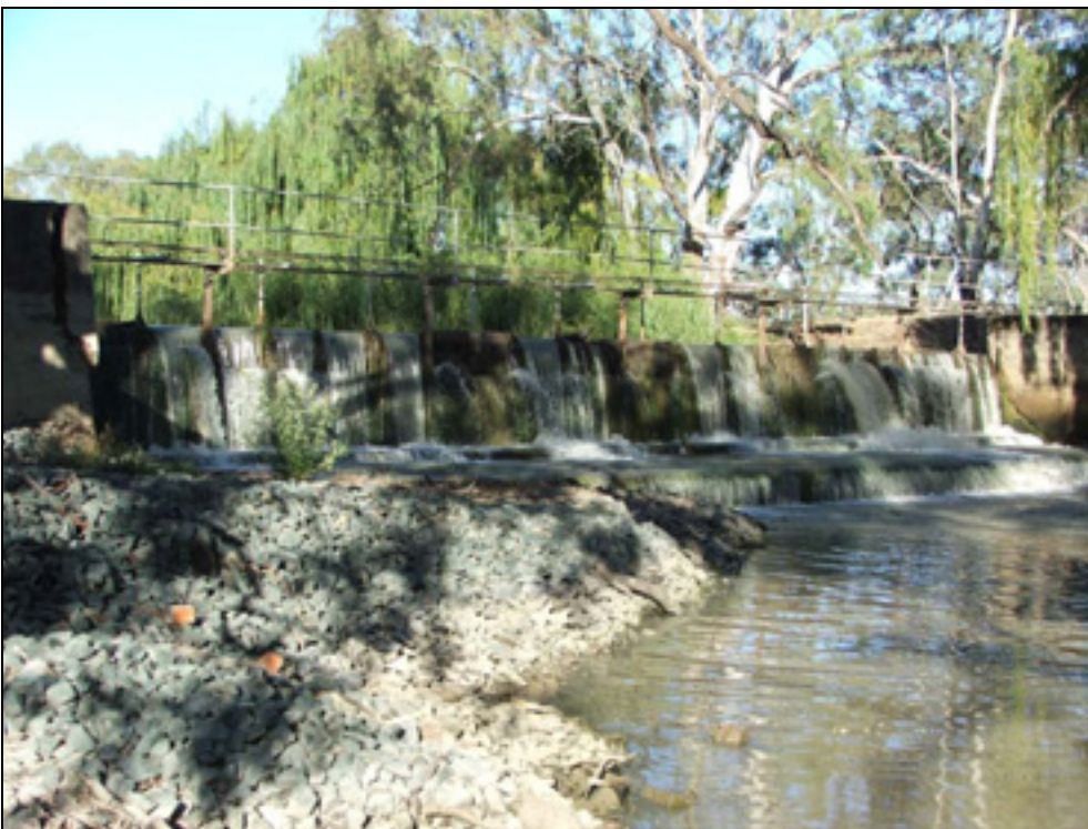
Figure 2. Hartwood Weir downstream erosion protection works, Billabong Creek (04.03.2005, 142ML/day).
