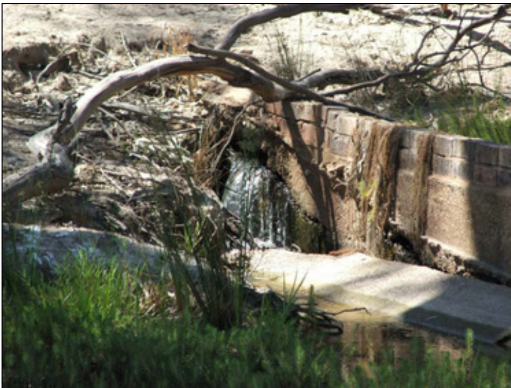
Figure 2. Widgee Weir structural failure on right hand side, Wakool River (02.03.2005, 42ML/day).
