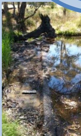
Obley Weir – restricting access for fish to upstream habitat.
