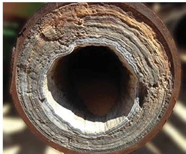
Figure 5. Scale build-up inside a pipe.
