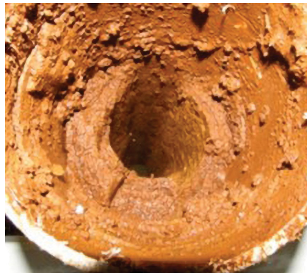
Figure 11. Iron and iron-loving bacteria blocking an irrigation pipe. Photo: Water Well Solutions .
