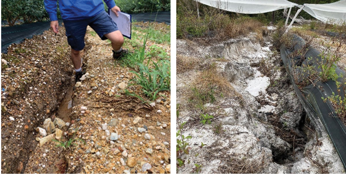
Figure 3. Washouts on a blueberry farm caused by intense rainfall.
