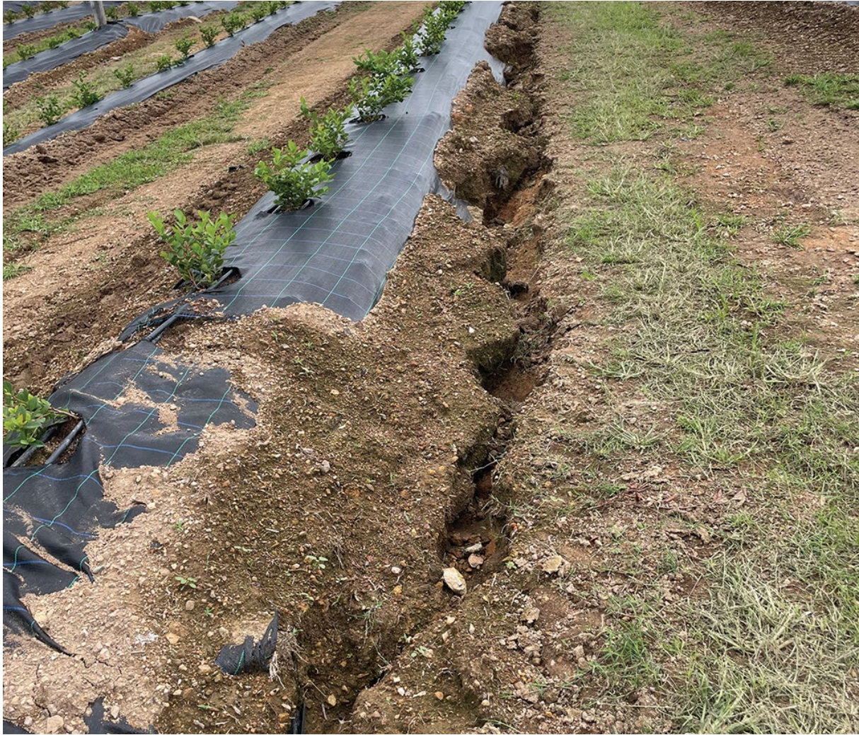
Figure 11. Scouring down the side of blueberry mounds after rainfall where ground cover was not established.
