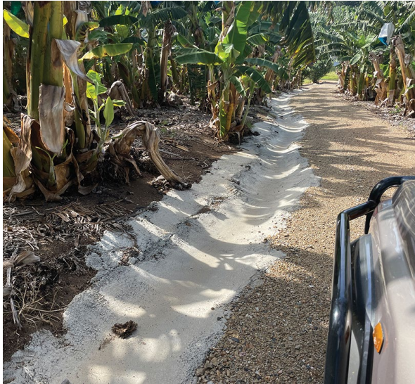
Figure 25. A concrete flume to divert water away from vulnerable slopes.
