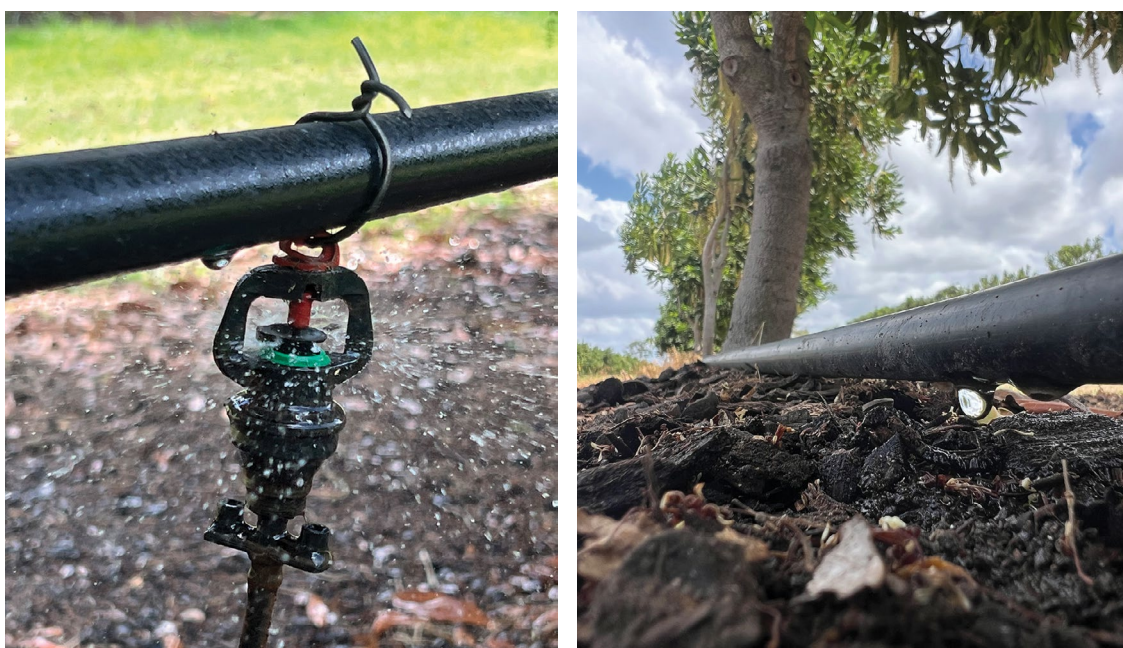
Figure 35. Mini-sprinkler (left) and dripper (right). Photos: Chris Fuller, Nutworks.
