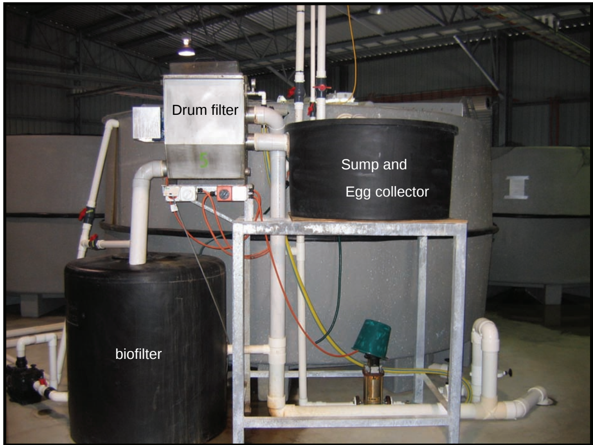
FIGURE 56: Controlled environment recirculation tank for broodstock maintenance at PSFI. Note the plumbing from the pump goes to an outdoor heater/chiller unit and then returns to the tank.
